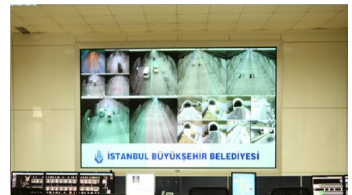
Tunnel Control Centre
