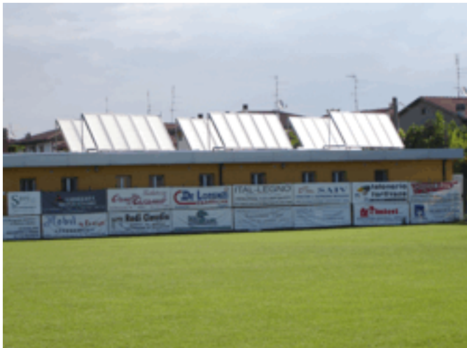
Solar thermal plant
